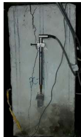
(ii) Pre-damaged PC column
