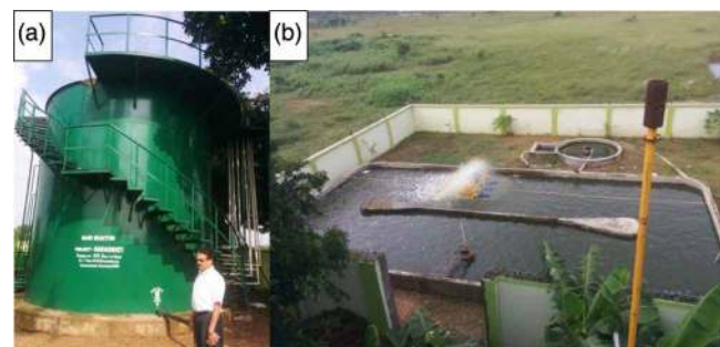
Figure 1 | (a) UASB reactor, (b) HRAP.
